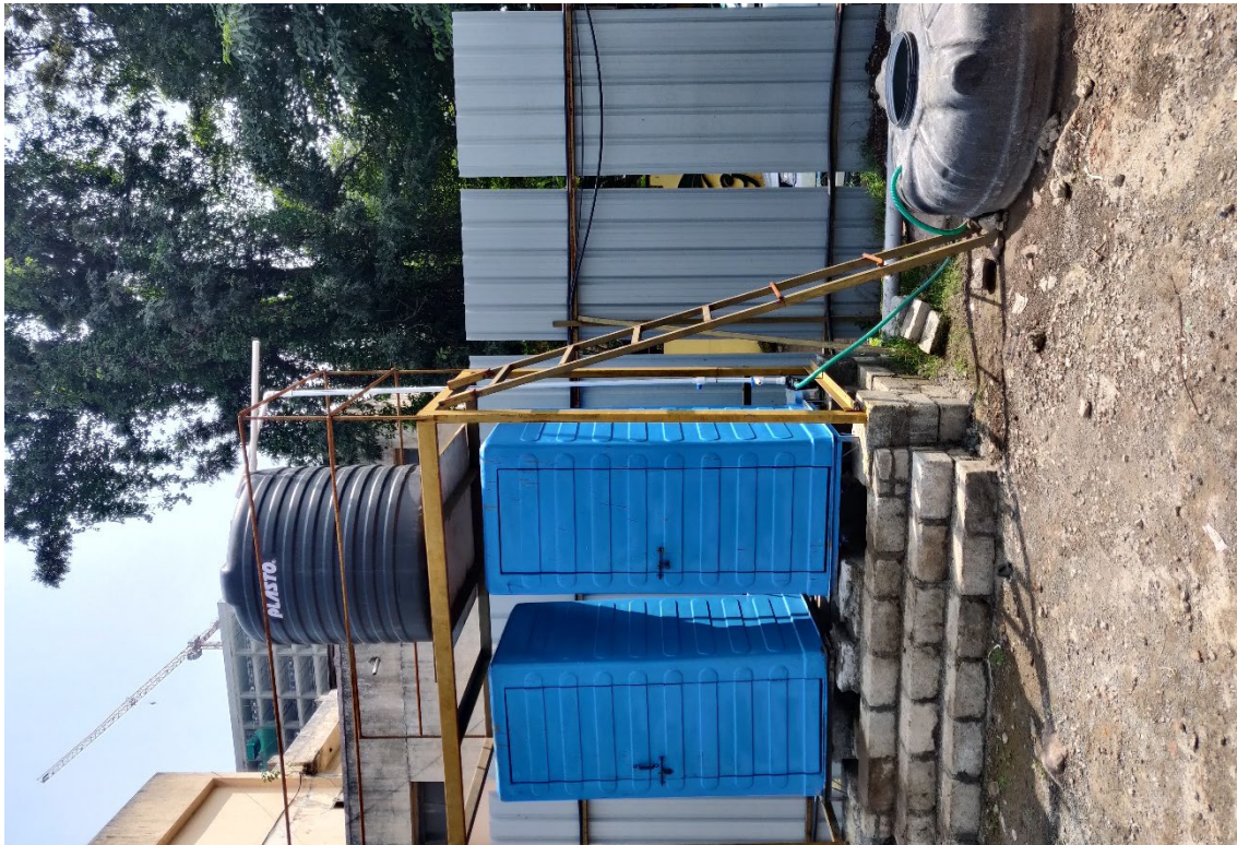
LABOR TOILETS FACILITY
